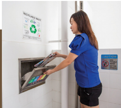
SEPARATE CHUTES FOR RECYCLABLE WASTE
