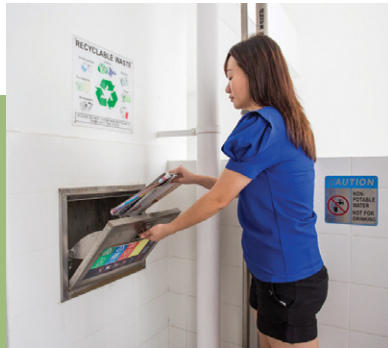
SEPARATE CHUTES FOR RECYCLABLE WASTE
