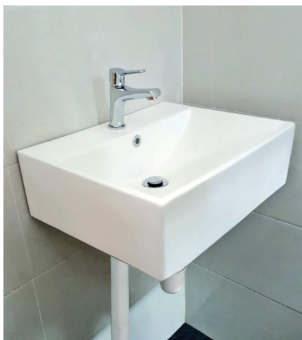
Wash basin with tap mixer
