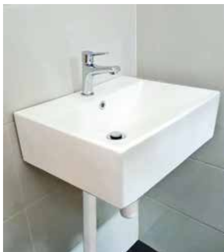
Wash basin with tap mixer
