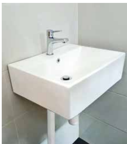
Wash basin with tap mixer
