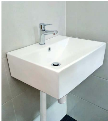
Wash basin with tap mixer
