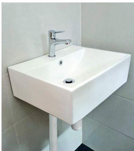
Wash basin with tap mixer
