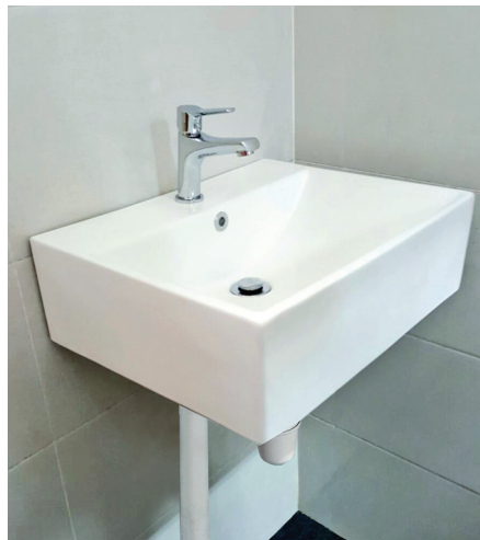
Wash basin with tap mixer
