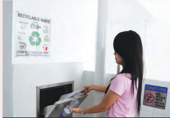
Separate chutes for recyclable waste
