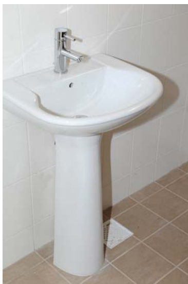
Wash basin with tap mixer
